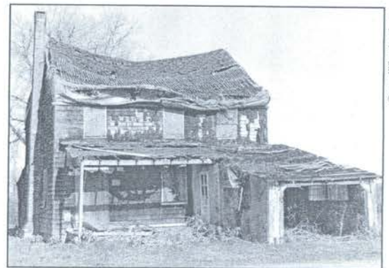
Near collapse, this State-owned 18th century farmstead was witness to the Battle of Monmouth.
