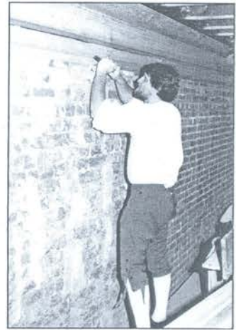
A costumed craftsman works on the restoration of the Courthouse at Colonial Williamsburg, where historic preservation is an integral part of interpretation programs.
