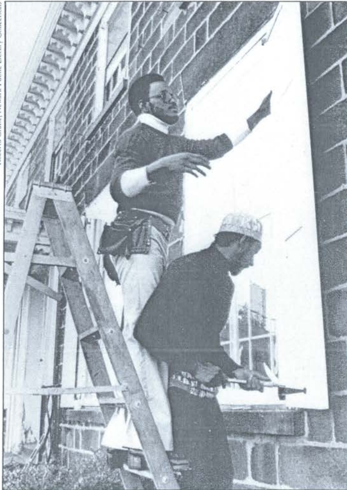
Restoration of Plume House, one of Newark's two remaining eighteenth century buildings.
