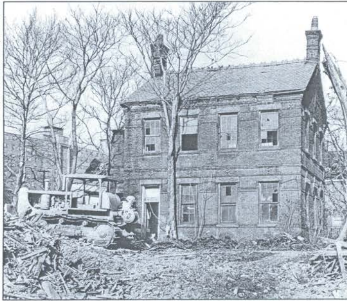
Newark laboratory of celebrated inventor and manufacturer Edward Weston, moments before its demolition in 1965.
