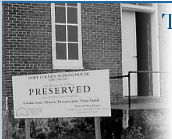
A program sign announces that restoration work is under way at the Port Colden School, Warren County.
